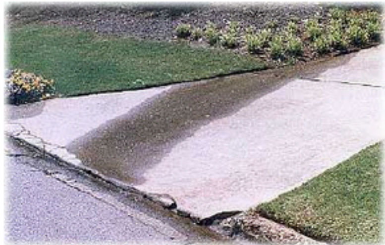
Ground water seeps to the surface the day after a storm.
